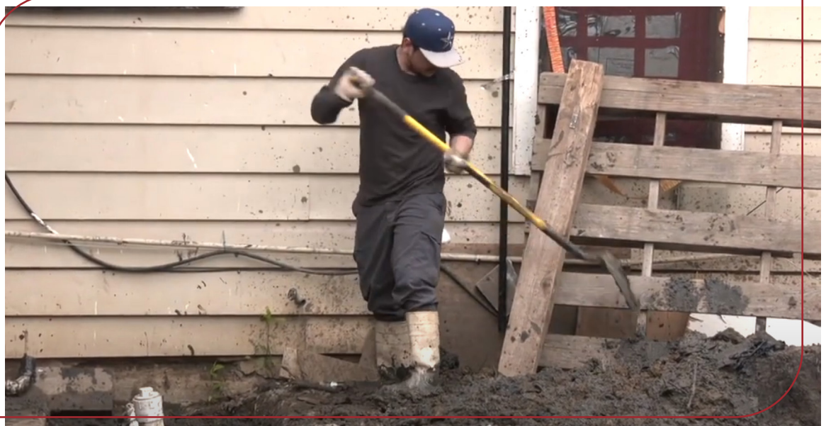
A repair in progress as part of the Fort Worth Priority Repair Program. Source: Neighborhood Services Department
