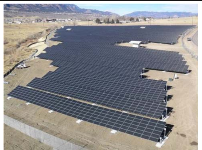
A PV System on a closed landfill near Atlanta Georgia. Source: Feasibility Study of Economics and Performance of Solar Photovoltaics at the Vincent Mullins Landfill in Tucson, AZ.
