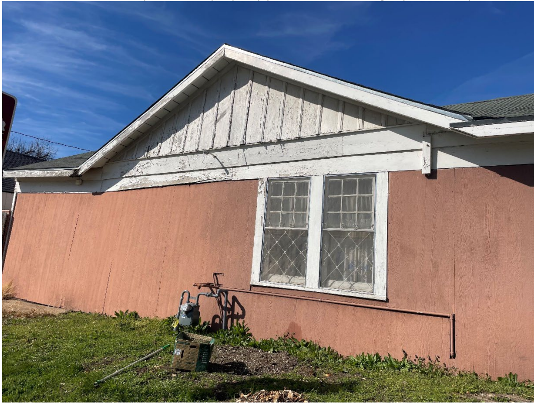
Pictures of the accessory structure property prior to demo, Images provided by HCLC staff
