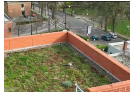
Green roof on Hamilton Apartments, Portland, Oregon, owned by the Housing Authority of Portland.
