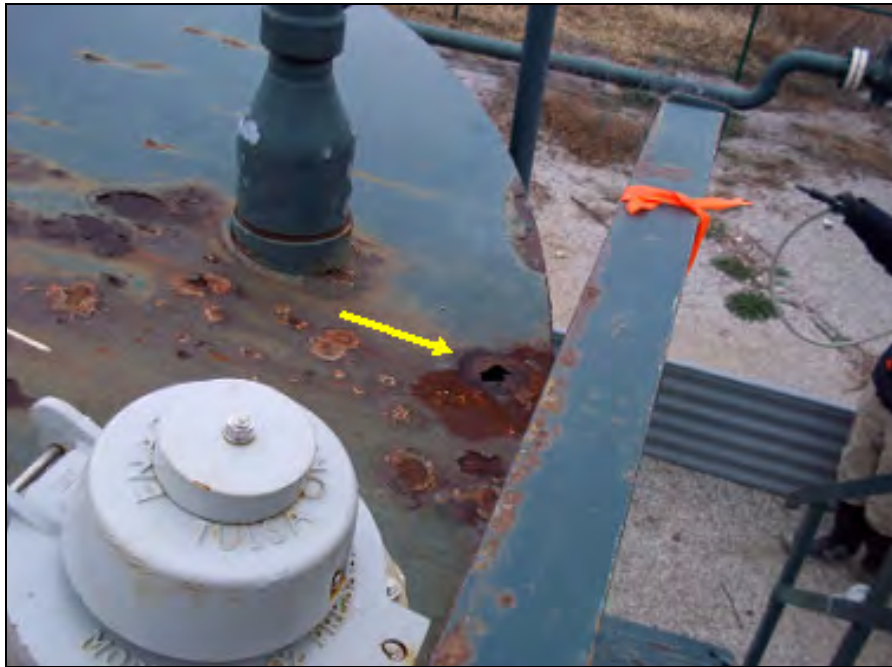
Figure 3.7-5. Hole in Tank Roof - Miscellaneous Emission Source
