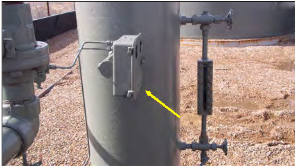
Figure 3.7-2. Pneumatic Valve Controller on Separator
