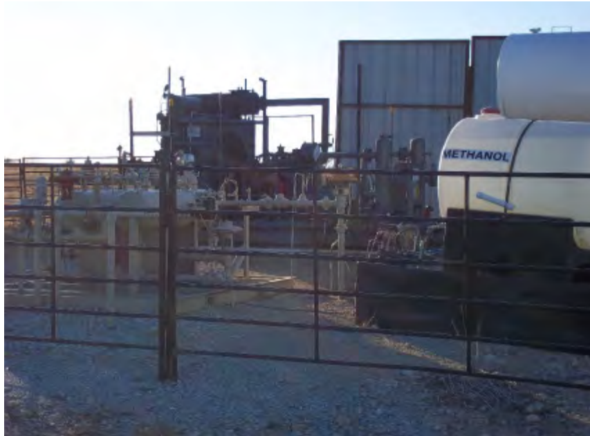
Figure 3.3-7. Site Documentation – Lift Compressor
