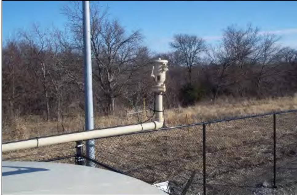
Figure 3.7-3. Storage Tank Vent
