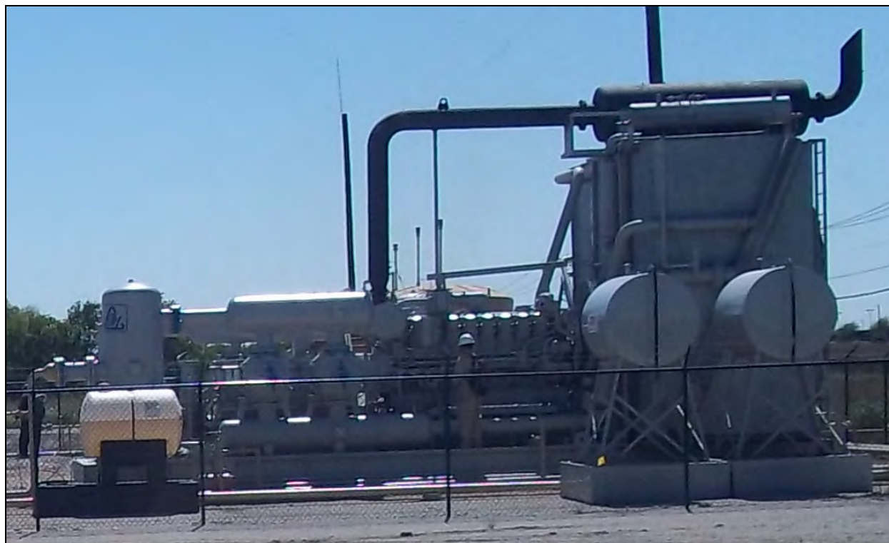
Figure 4.1-3. Natural Gas Compression Engine
