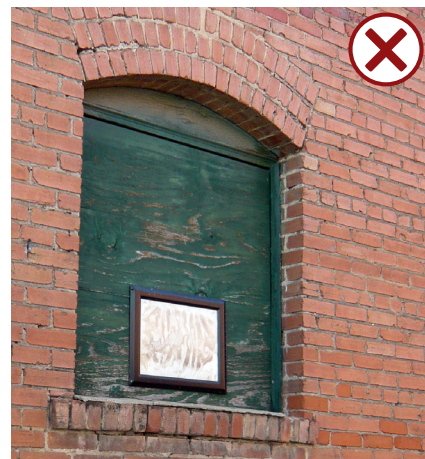
Restore a historic window opening that has been altered. For example, this opening has been blocked. Restoring the window is best practice in this situation.
