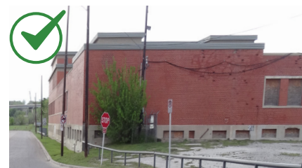
Simplicity in building form or material can be a key character-defining feature.
