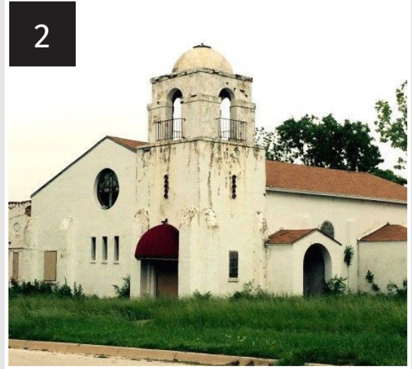
Once scheduled for demolition the building was not maintained and was left abandoned and dilapidated.
