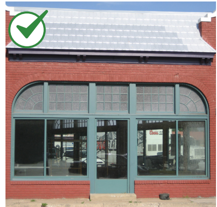
Retain historic coatings such as paint that help protect exterior materials from moisture and ultraviolet light.
