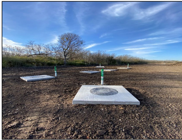
Source: Dannenbaum Engineering Corp's Site Observation Report - January 14, 2021
