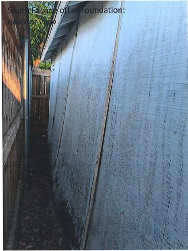
Damage at base: Open to the elements.
